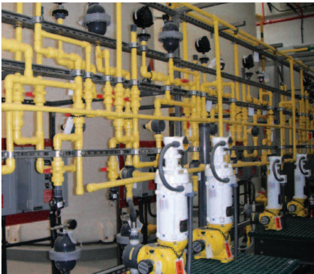
This caustic storage and metering system at New Design Plant Two is one of 10 chemical storage and metering systems found at the new chemical residuals facility.
