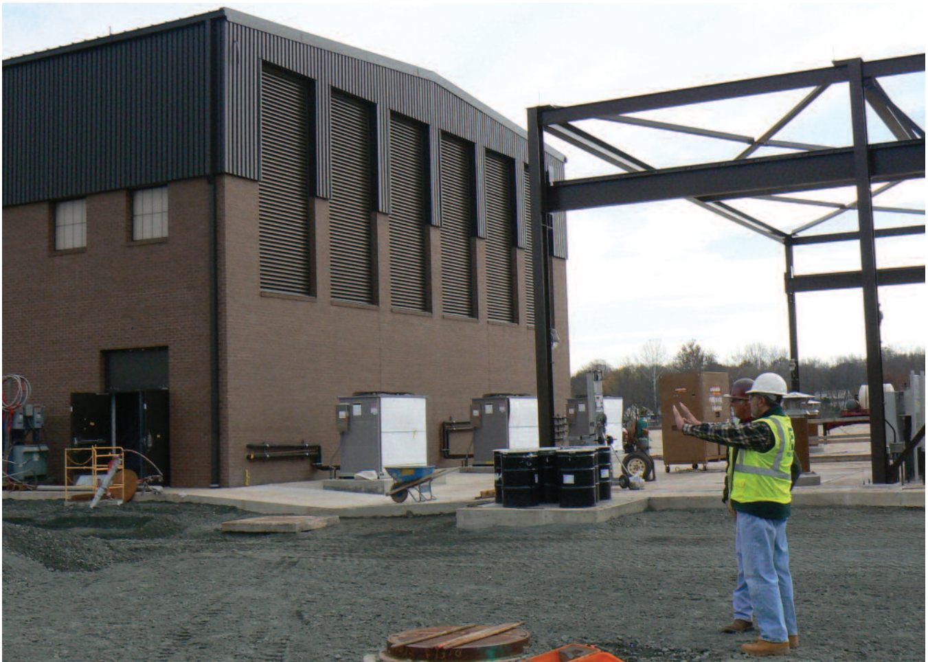
Fru-Con Project Director Osama Madkour (foreground) confers with Fru-Con Mechanical Superintendent Ron Jenkins about upcoming work for the electrical building and pump station at the Flat Branch Pump Station & Force Main Improvement project in Manassas, Virginia.
