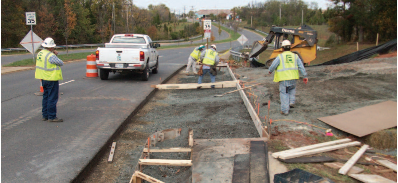
Fru-Con workers prepare to place the concrete apron at the entrance to the Winters Branch Pump Station off Godwin Drive in Manassas, Virginia.
