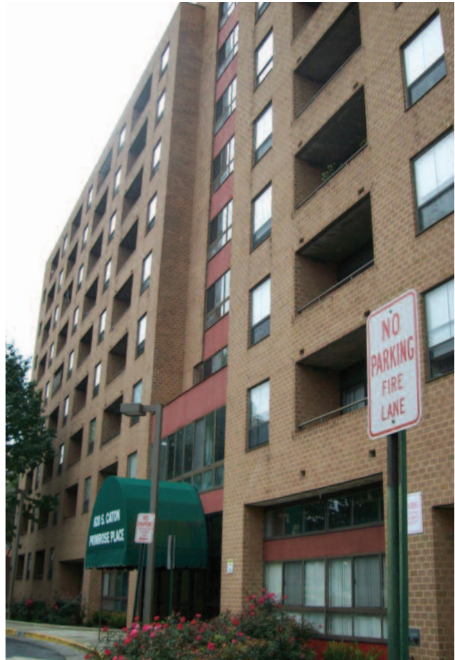
Centennial is waterproofing and tuck-pointing the 12-story façade of Baltimore's Primrose Place. All exterior windows are being replaced with energy-efficient alternatives.
