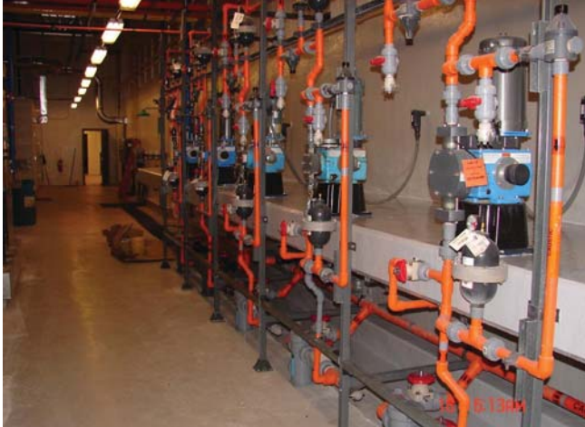
As water from the Potomac River enters the plant, this series of new chemical feed pumps initiates preliminary treatment with sodium hydroxide and zinc orthophosphate to jumpstart the purification process.
