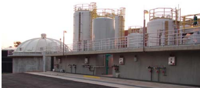
The western side of the campus features a series of circular chemical storage tanks housing the sodium hydroxide, sodium hypochlorite, ferric chloride and zinc orthophosphate used in water purification. The domed structure (left) houses the sludge gravity thickener, where raw water is separated from sludge early in the cleansing process.
