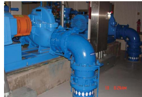
Fru-Con crews upgraded the plant's horizontal split case centrifugal pumps with two new 400-horsepower units that increase the plant's processing capability. The two pumps alternate in low demand and simultaneously meet peak demand requirements.
