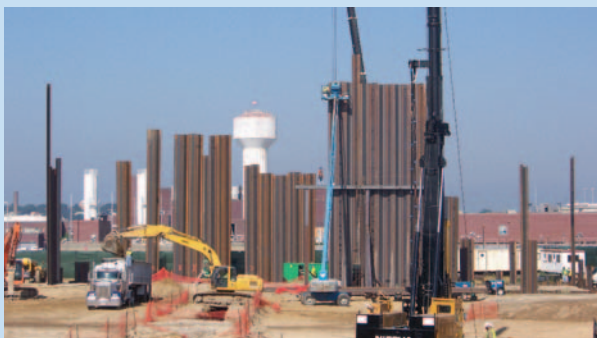
Fru-Con Construction crews mobilized in November 2009 to begin work on the world's largest fixed-film denitrification system, part of Fru-Con's $116 million expansion of Patapsco Wastewater Treatment Plant in Baltimore, Maryland. See story on page 4.
