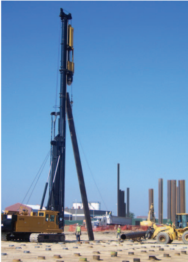
Pile driving operations are under way at Baltimore’s Patapsco Wastewater Treatment Plant.
