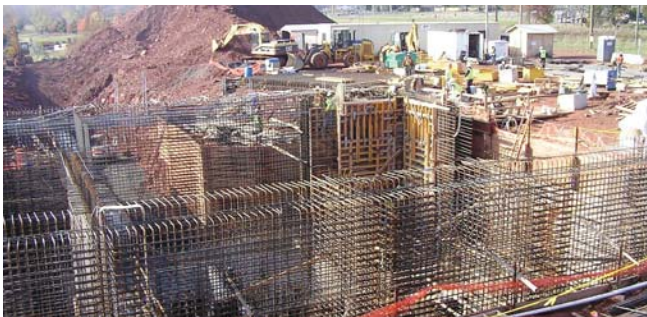
At 10 months into the project, Fru-Con Construction is ahead of schedule on its $39.4 million assignment at the Flat Branch Pump Station in Manassas, Virginia.
