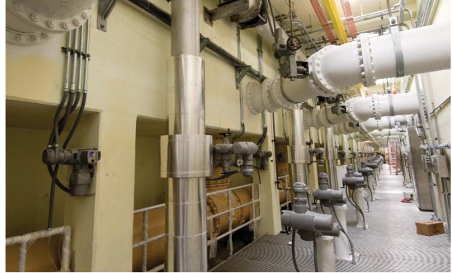
The Arlington County facility can now process 40 million gallons of wastewater per day, a 33 percent increase in capacity.
