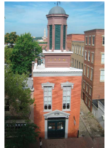
The Centennial team expertly restored the cupola of the Friendship Fire Company firehouse, built in 1855.
