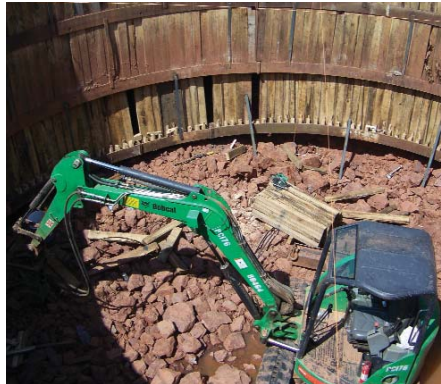
Fru-Con's $39 million Flat Branch Pump Station & Force Main Improvements project includes constructing a shaft with a shoring system to facilitate a tunneling machine for installation of a 36-inch raw sewage line.
