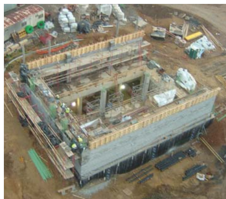
Fru-Con developed custom soil engineering solutions to address the specific geological condition found beneath the footprint of every new building at New Design.
