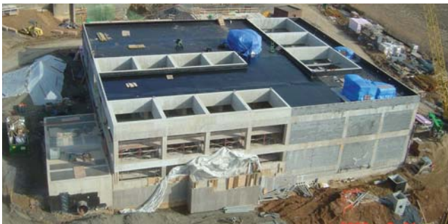
Five new buildings are being constructed at New Design. The expansion will nearly triple plant capacity to 25 million gallons per day.
