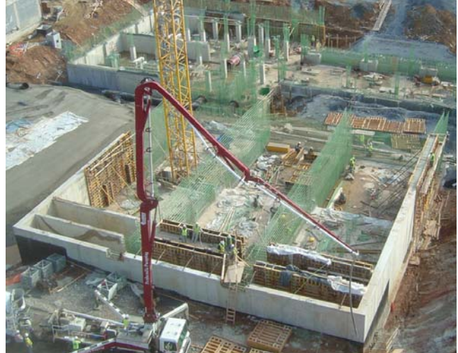
Fru-Con is on pace to complete placement of the 23,000 cubic yards of concrete needed at New Design in July.
